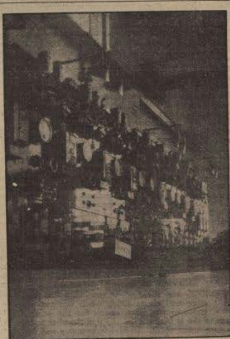
The Power House Switchboard at Brookmans Park.
